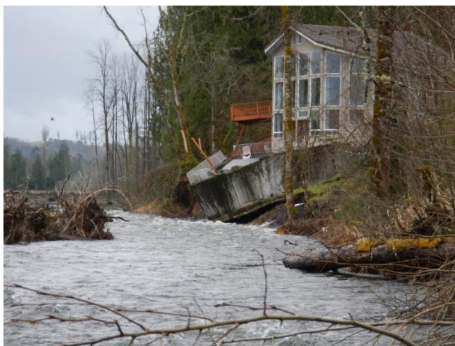
Figure 3.3. Damage from Channel Migration
