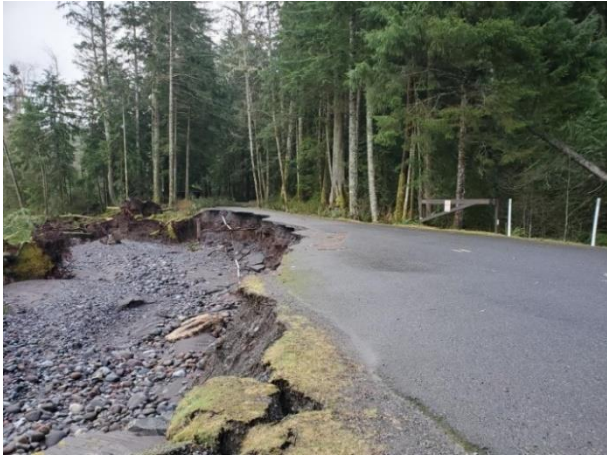
Figure 6.78. Looking Upstream at the Upper Carbon River Washout Area
