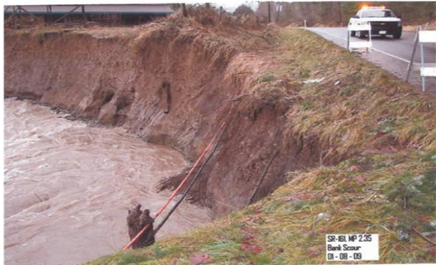
Figure 6.101. Left Bank Scour along SR 161, RM 5.2–5.3
