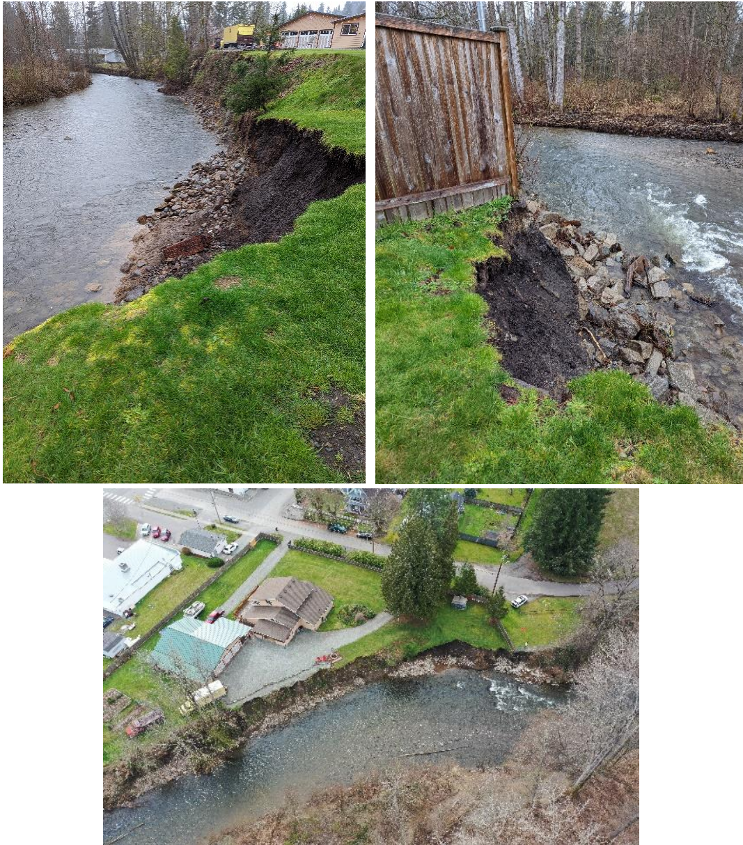
Figure 6.85. Bank Erosion Impacting South Prairie Wastewater Treatment Plant Outfall, 2022
