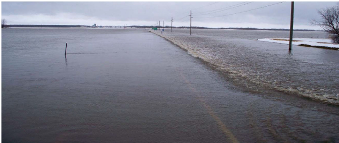
Figure 4-4. Photograph of Roadway Flood Overtopping 52
