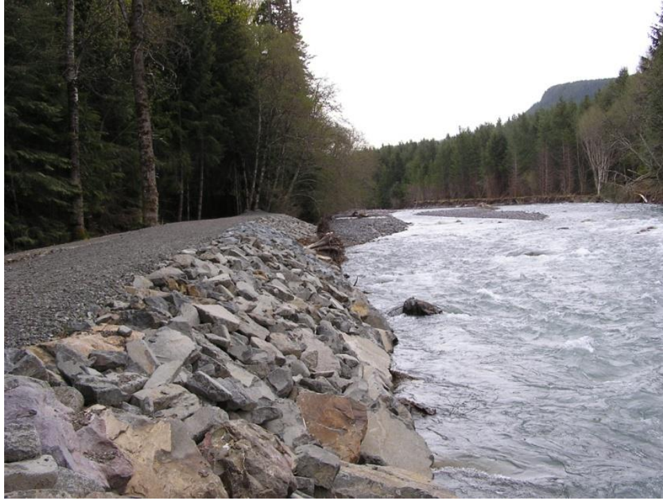
Figure 6.57. RM 46.2 Right Bank Levee at 583rd Avenue East along the White River
