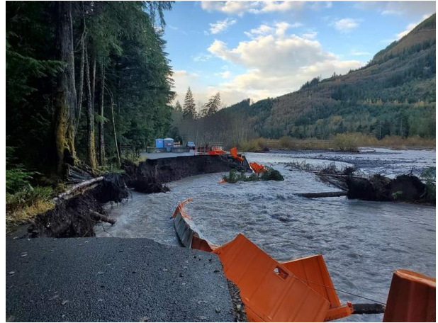
Figure 6.79. Looking Downstream at Lower Carbon River Washout Area
