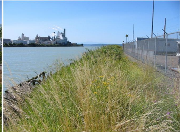
Figure 6.9. Right Bank Revetment at Port of Tacoma Downstream of East 11th Street (looking downstream)
